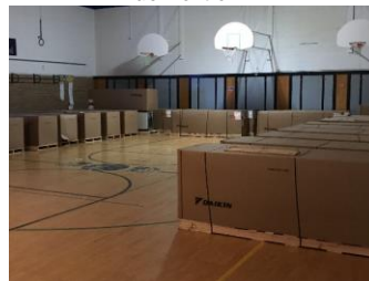
Unit ventilators delivered at Chestnut Hill
